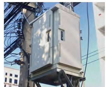
Internet Control Box
