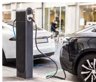
EV Charging Stations
